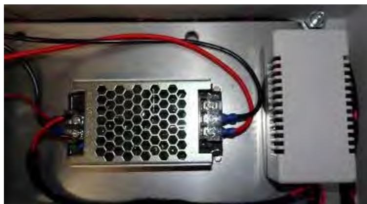
Figure 12: 24 VDC auxiliary power supply
