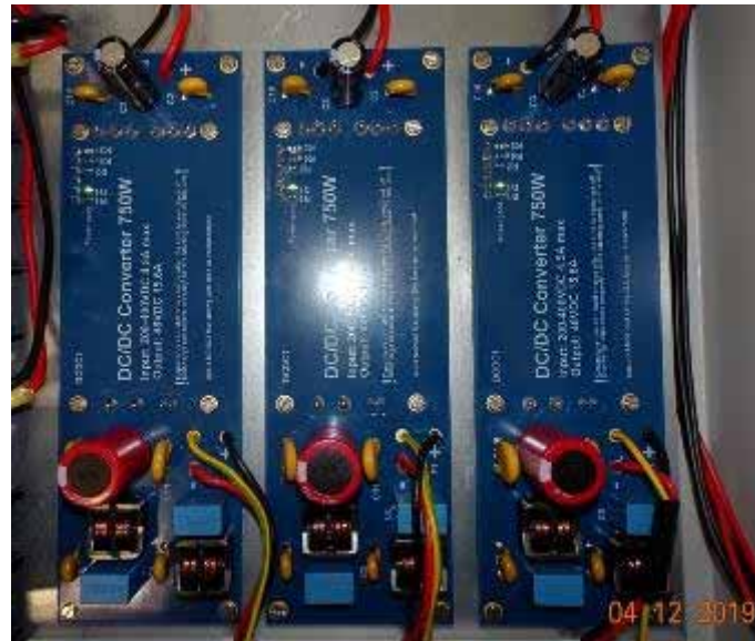
Figure 9: three DC/DC converters
