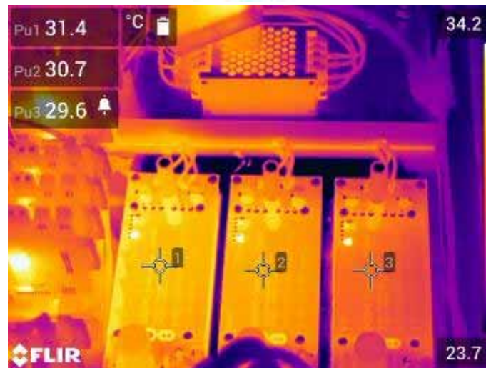
Figure 11: Infrared image of DC/DC converters in idle state
