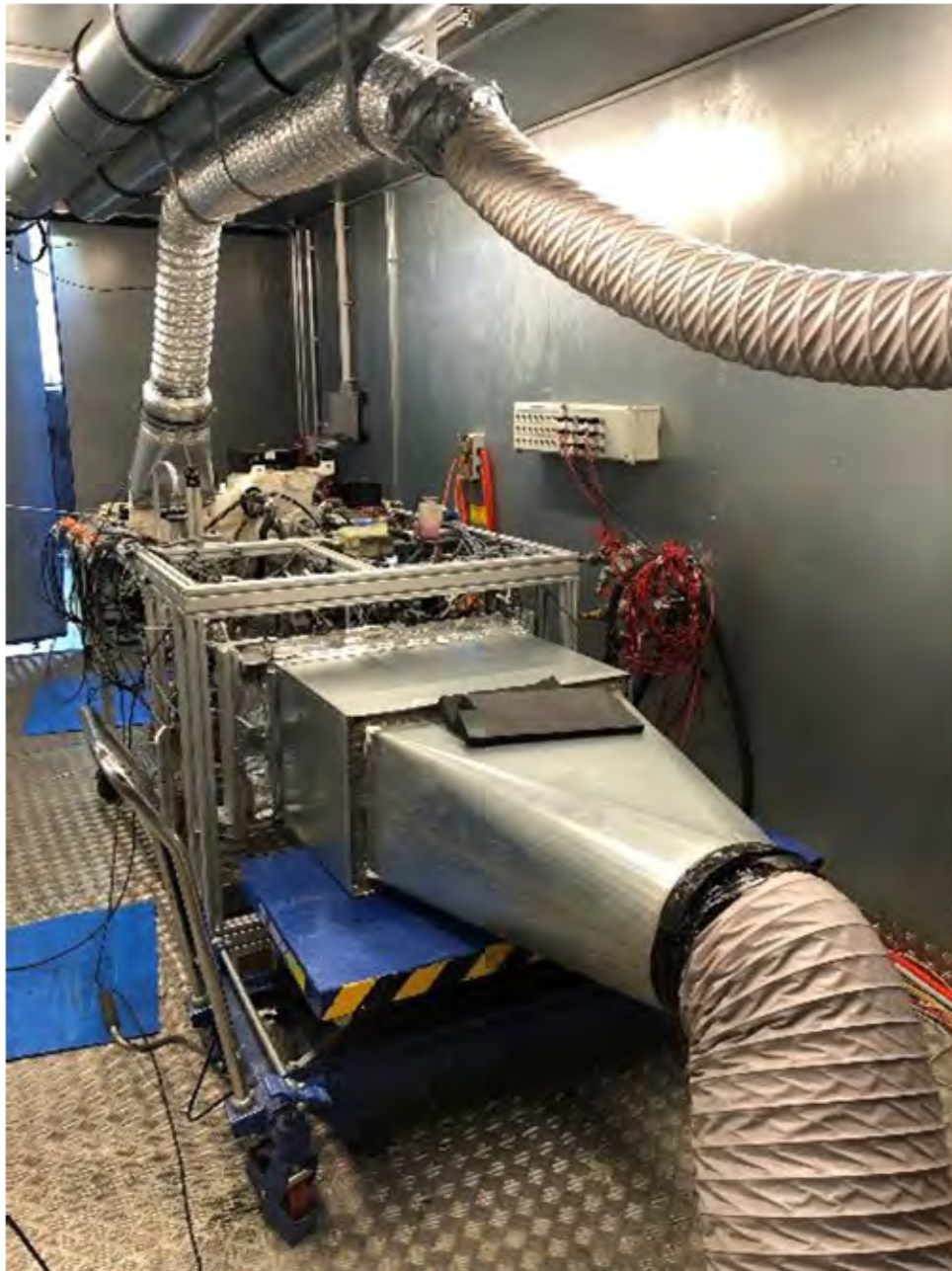
Figure 66: Build-up and instrumentation of Step-2 (entire VTMS) at AC system testbed
