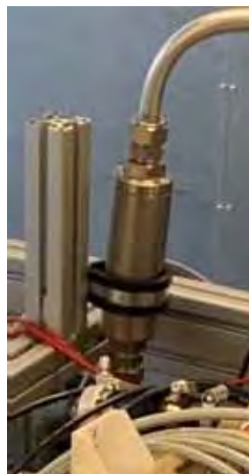
Figure 57: Refrigerant filter installed before the compressor on testbed
